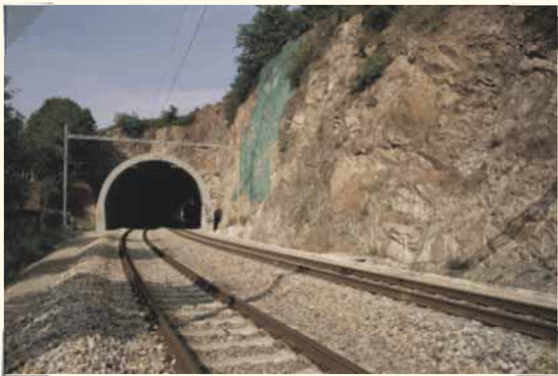
Optimalizace trati Brno-Skalice nad Svitavou, tunel č. 1, Brno-Obřany Optimising of Brno-Skalice nad Svitavou railway track, tunnel no. 1, Brno-Obřany
