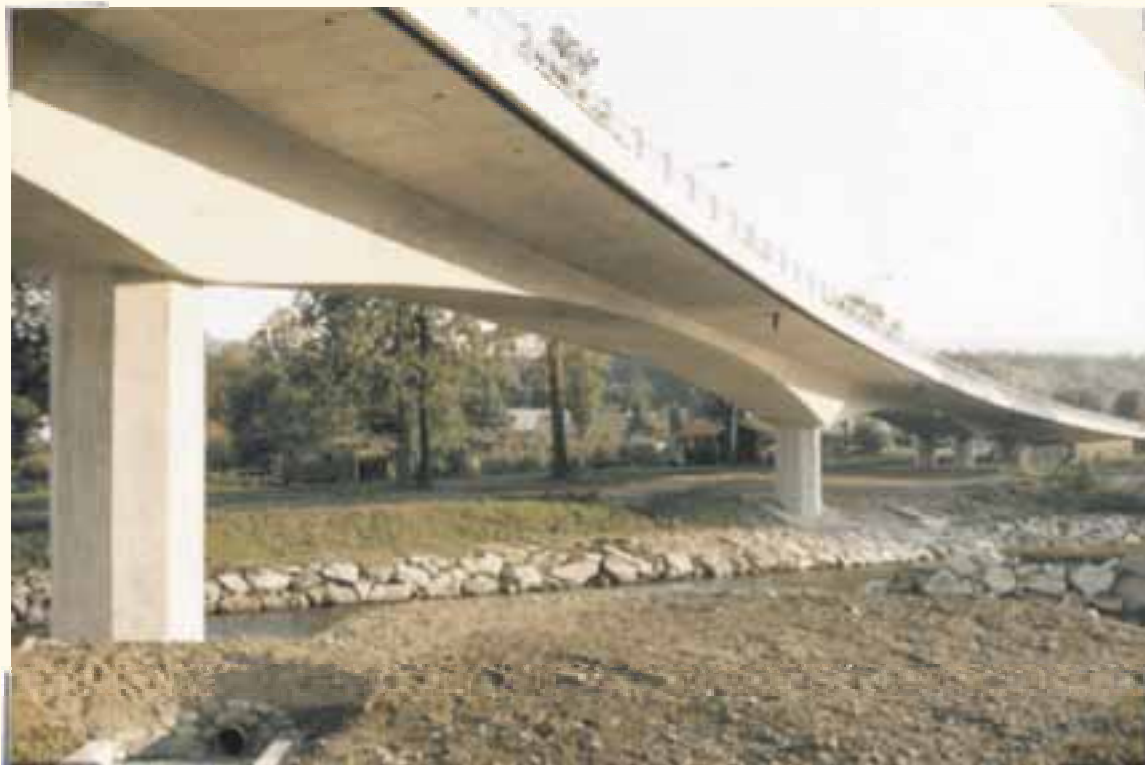
Novostavba silnice I/44, Mikulovice obchvat Construction of the I/44 road, Mikulovice bypass
